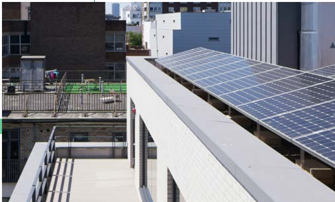
Reducing carbon intensity at 160 Old Street, EC1 through the use of renewable energy using photovoltaic cells.
